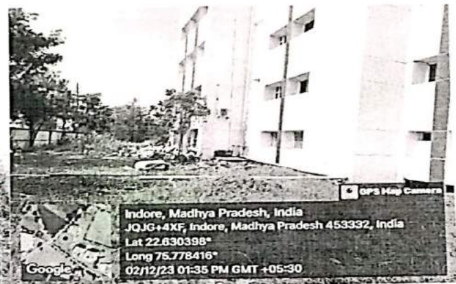
Rain water harvesting system: 02
